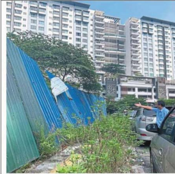
Yee at the junction of Jalan Vista Mutiara Satu ana Jalan 14/33B in Kepong Baru where the hoarding is falling apart.
