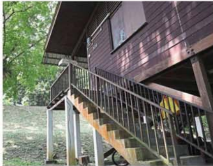
Wooden staff quarters built in the 1960s are still in good shape and are a part of FRIM's Unesco submission.
