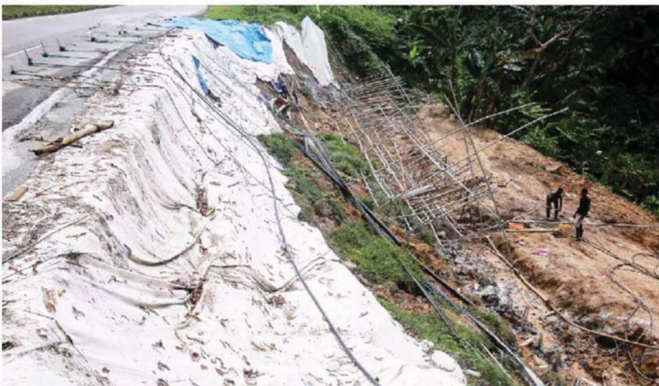
Workers in Seremban carry out works to stabilise a slope along Jalan Pesiaran Senawang 3 following a landslide which caused cracks to appear on the road. — Bernama photo
