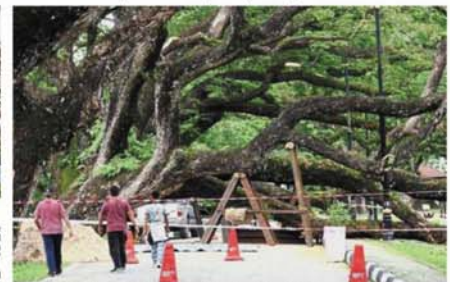
Clearing the road: Workers conducting repair work along the stretch of road where the rain tree fell at the Raintree Walk at Taiping Lake Gardens. — Bernama
