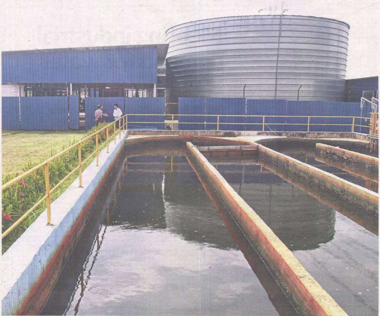
Treated for reuse: The Setia Alam water reclamation treatment plant is distributing water to industries nearby through underground pipelines. — Photo: SAM THAM/The Star
