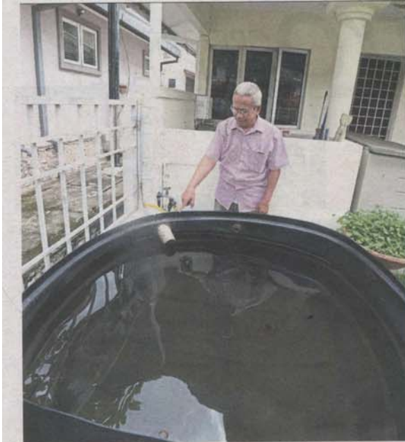
Syed has created his own rainwater harvesting system.
