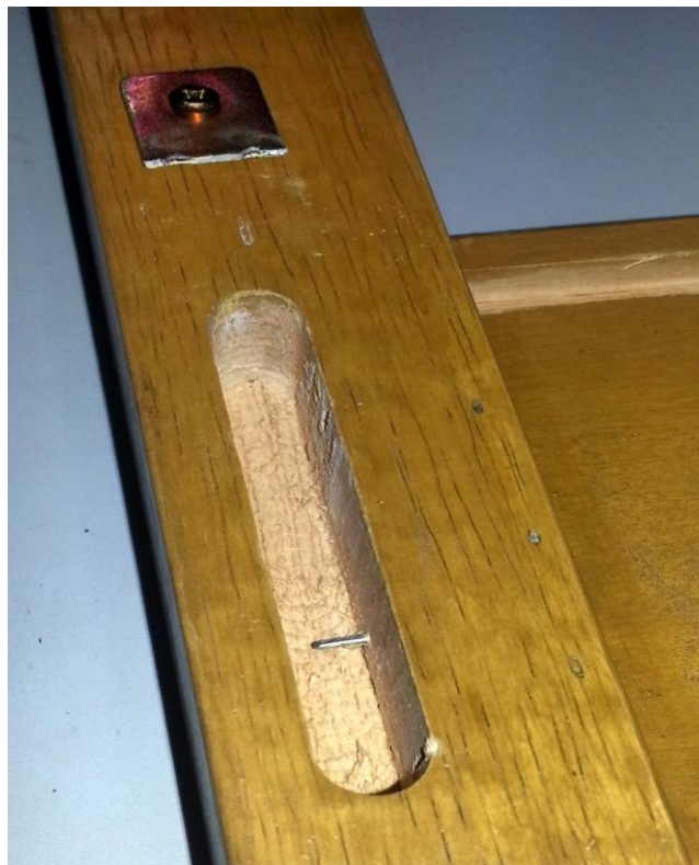
Figure 9 The application of nail or L-bracket does not provide significant support on the joint strength if the fundamentals of good mortise and tenon are not fulfilled
