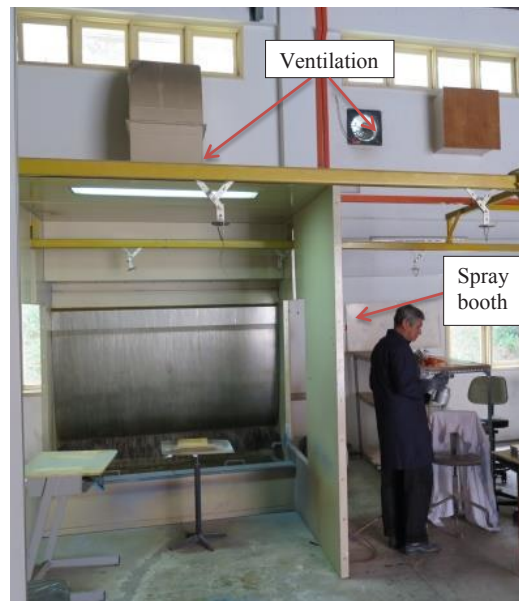
Figure 2 Ventilation and spray booth
